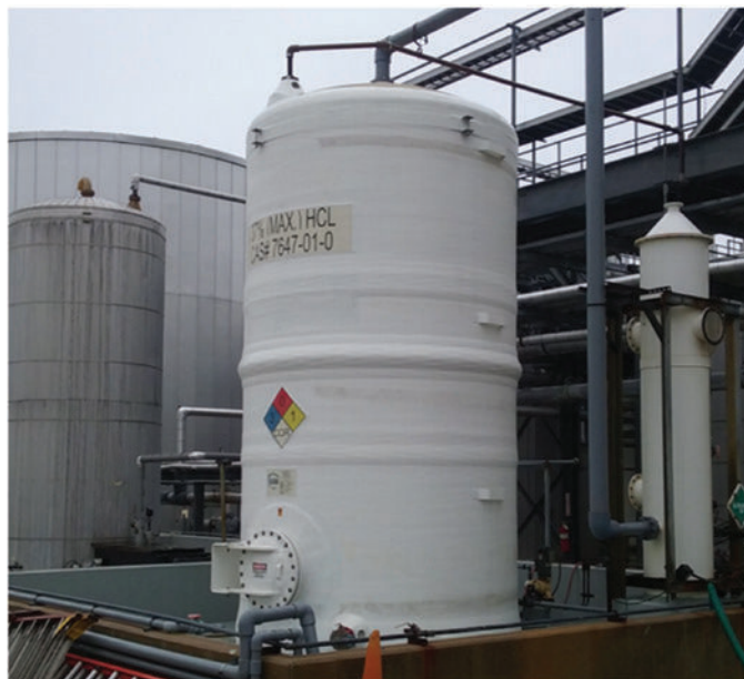
Figure 1. Hydrochloric acid tank.
