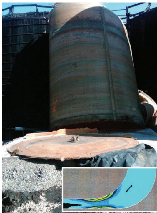
Figure 4. Catastrophic failure of acetic acid tank.
