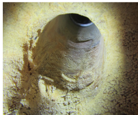
Figure 7. Tank drain damage.
