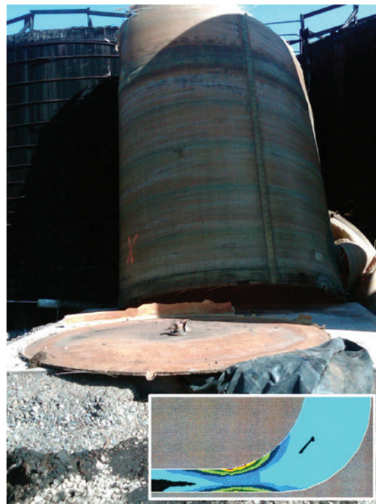
Figure 4. Catastrophic failure of acetic acid tank.
