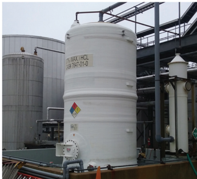
Figure 1. Hydrochloric acid tank.
