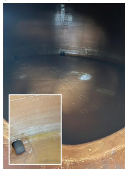
Figure 8. Damage to tank bottom, knuckle, and lower shell.
