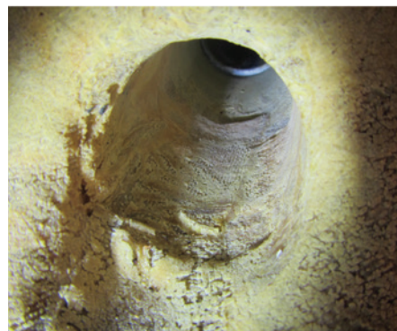
Figure 7. Tank drain damage.
